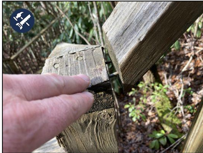
handrail is coming loose from its mount here...recommend repair
