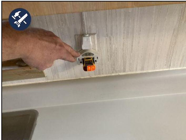
outlet next to kitchen sink is not a GFCI. This can be a shock hazard. Recommend replacement by electrical contractor
