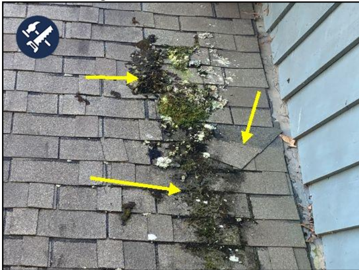
a shingle tab has slid down out of place. It does not appear to be leaking at this time...however it should be repaired by a roofing contractor. Also the moss growing here needs to be sprayed with fungicide.
