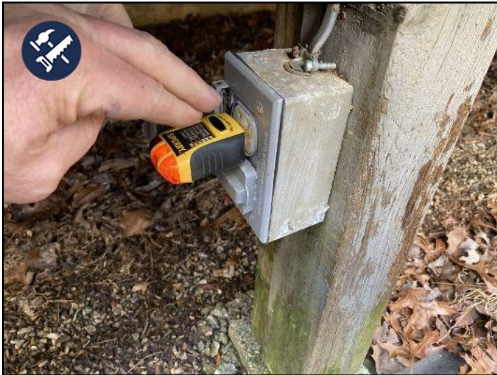
not GFCI protected.
