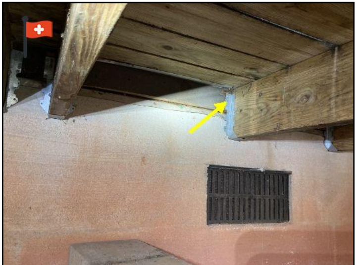
the deck is not properly attached to the home. Most deck failures occur at the attachment point at the house. The hangers for the joists are not fully bearing on the ledger. The ledger is not bolted or structurally screwed to the home. Recommend evaluation and repair by qualified contractor
