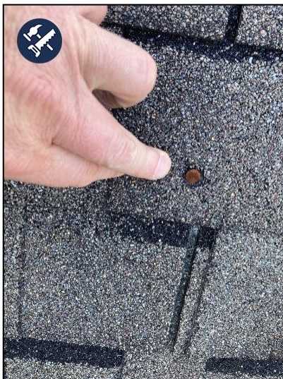
a nail in the exposure part of the shingle is not proper building practice. Recommend a dab of roofing cement over this nail head.
