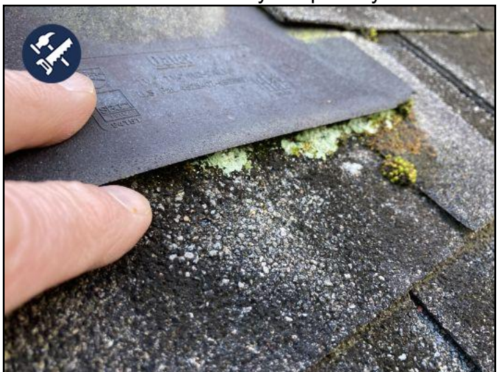
most of the mold is on the north facing parts of the roof
