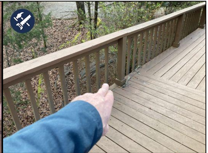
the hand rail on the deck...facing the front...south of the house...is loose and in need of reinforcement.
