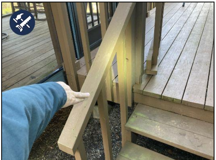
this handrail is loose at the rear deck. Recommend repair by qualified contractor
