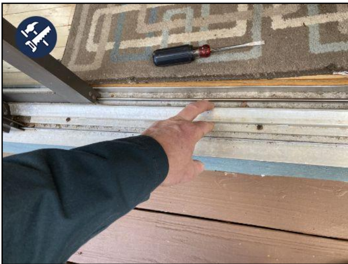
sliding glass door facing the back has a loose track/guide. The screws securing this are loose. Recommend repair.
