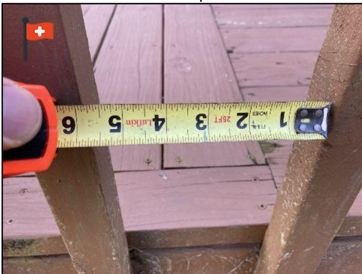
the balusters on the deck should not be more than 4 inches apart as to prevent a child from getting their head caught between them. While we are not code inspectors, we will still give the information and then let the parties involved decide on any action.
