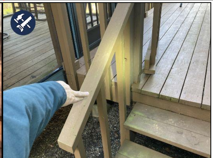
this handrail is loose at the rear deck. Recommend repair by qualified contractor
