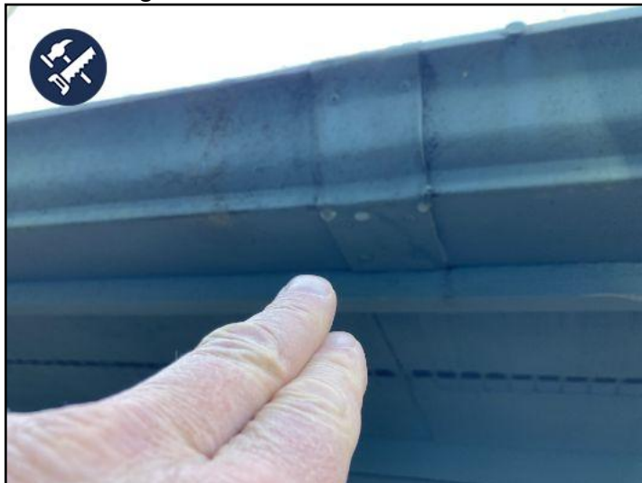
leaking gutter at the detached covered porch in the back. This is introducing moisture next to the deck. Recommend sealing with some gutter glue.
