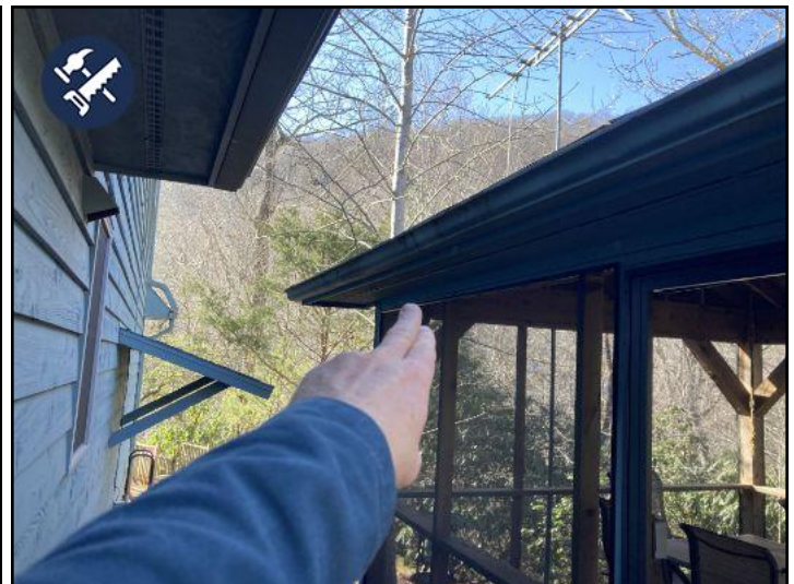
location of leaking gutter.
