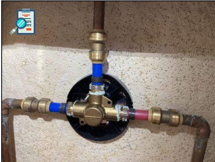
while the visible copper plumbing was in good shape...it will eventually fail. Unknown how long that could be....could be another 30 years.
