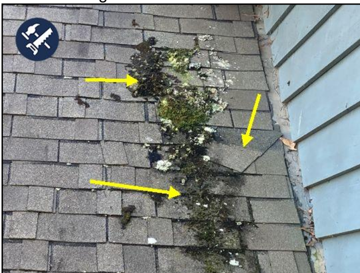
a shingle tab has slid down out of place. It does not appear to be leaking at this time...however it should be repaired by a roofing contractor. Also the moss growing here needs to be sprayed with fungicide.
