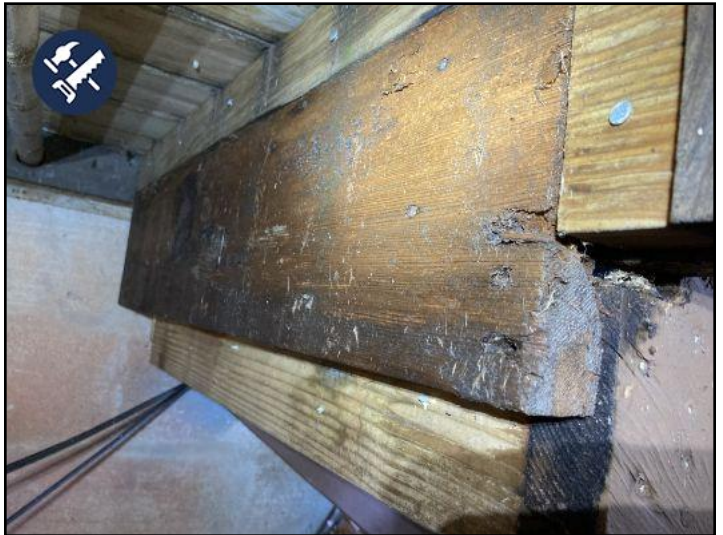
This ledger board for the rear deck steps (next to a/c compressors) is very wet and is rotting/soft. This needs to be replaced by a qualified contractor.
