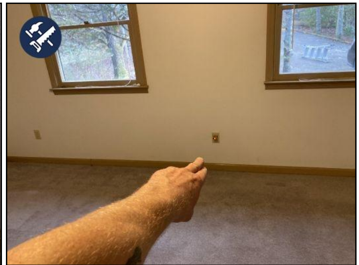
this outlet in the first floor bedroom is not grounded. This is the only one in the house...indicating to me that the receptacle itself was miswired or is defective. Recommend replacement
