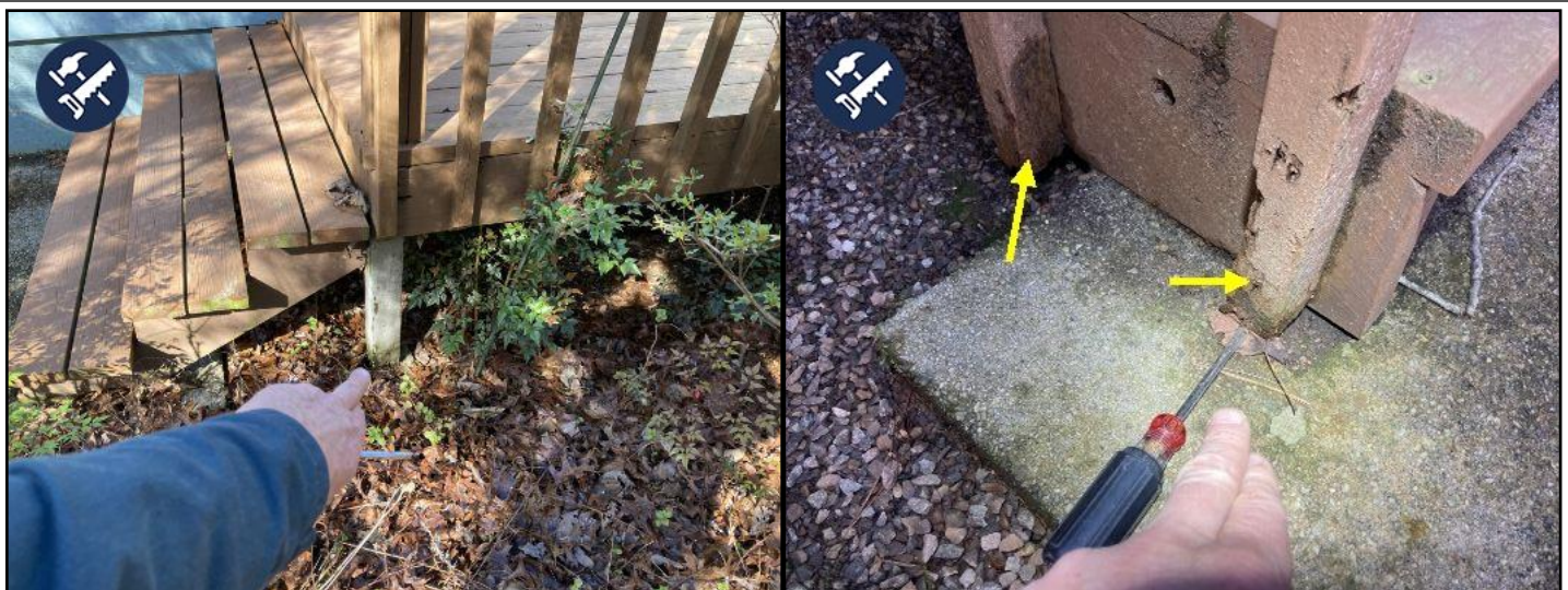
at the steps to the rear deck nearby the a/c compressors....there is rotted wood at the balusters. This handrail is also loose and in need of reinforcement.
