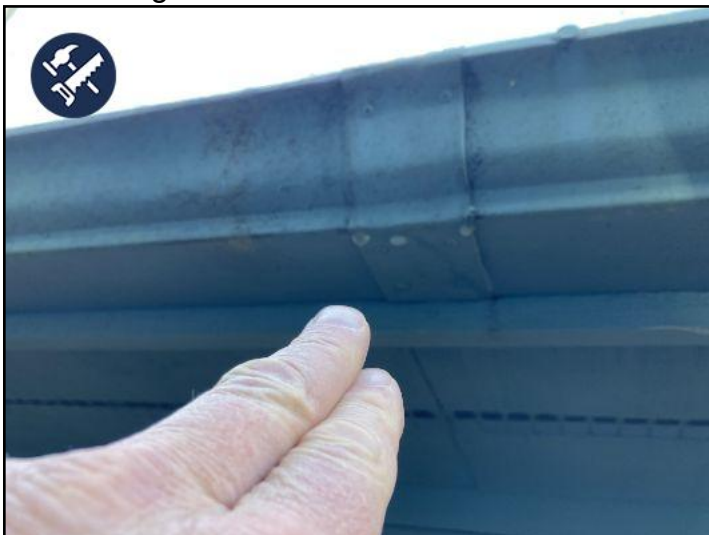
leaking gutter at the detached covered porch in the back. This is introducing moisture next to the deck. Recommend sealing with some gutter glue.
