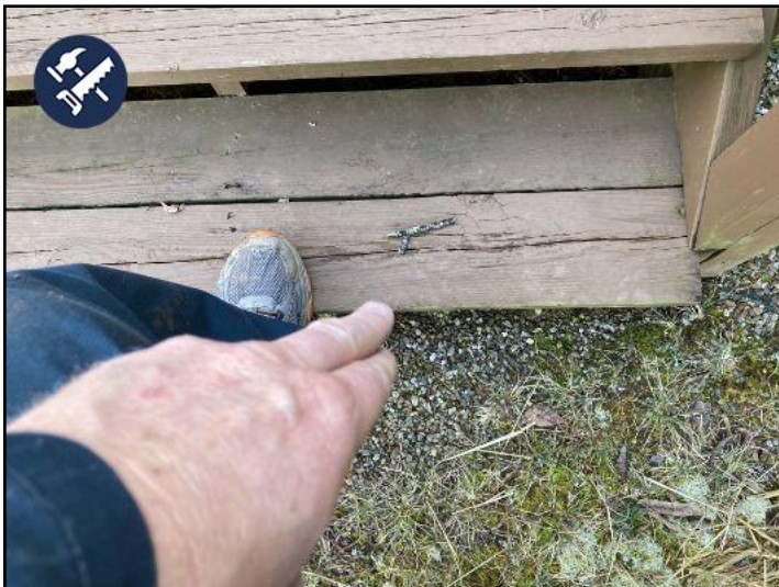
this bottom step off the rear deck...out to the back yard....is cracked and beginning to fail. Recommend replacement.
