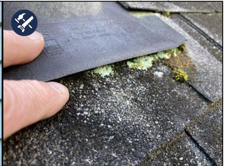
most of the mold is on the north facing parts of the roof
