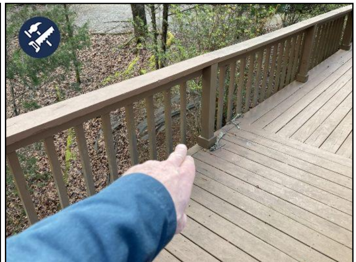
the hand rail on the deck...facing the front...south of the house...is loose and in need of reinforcement.
