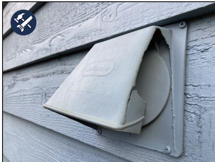
the upstairs bathroom vent is damaged. Recommend replacement.
