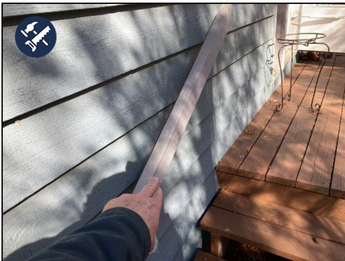
handrail at front entry steps is loose. Recommend repair.
