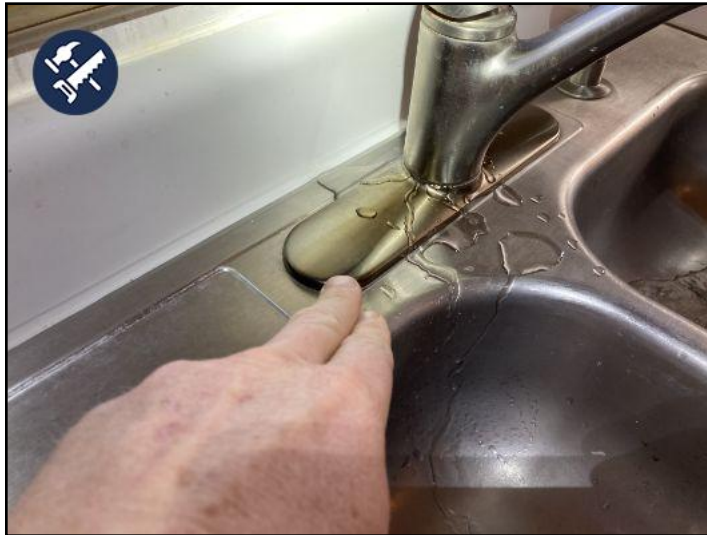
kitchen sink faucet leaks. Recommend replacment by plumbing contractor
