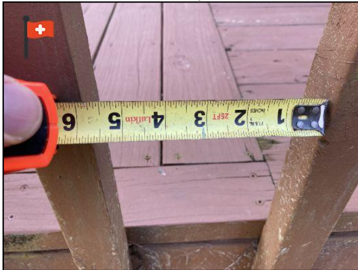
the balusters on the deck should not be more than 4 inches apart as to prevent a child from getting their head caught between them. While we are not code inspectors, we will still give the information and then let the parties involved decide on any action.
