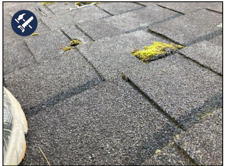
moss on the roof will shorten an asphalt shingles lifepan. Recommend spraying a fungicide on the affected areas every couple of years.
