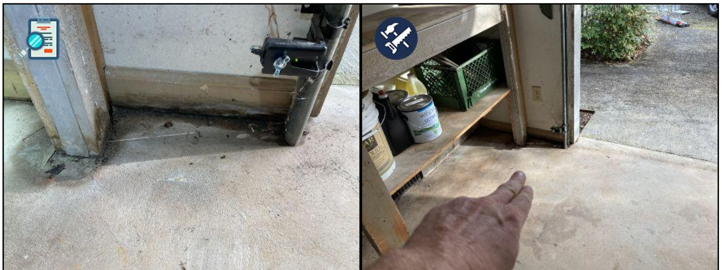
some water staining next to garage door...is not wet currently and wood is still structurally fine...monitor for possible water issues
