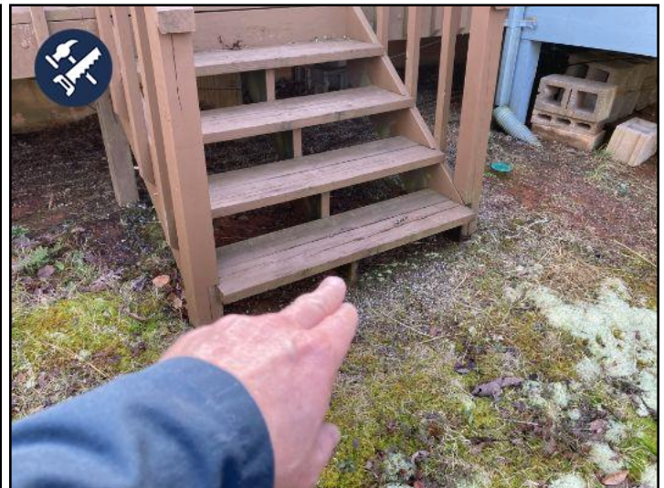
location of deteriorated step.
