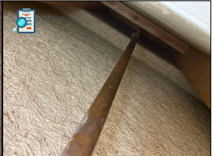
copper plumbing throughout the home. Copper has a life span and will eventually wear out/corrode and leak. Recommend budgeting for complete removal of all copper and replacement with pex.
