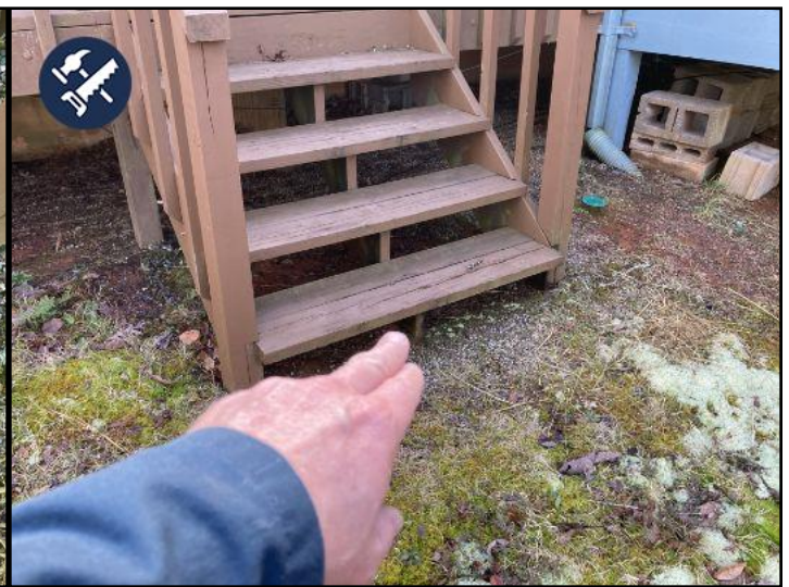
location of deteriorated step.
