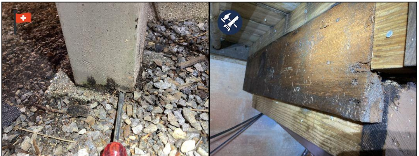
another 4x4 post that is beginning to rot from water exposure/contact with concrete footer.
