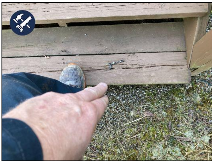
this bottom step off the rear deck...out to the back yard...is cracked and beginning to fail. Recommend replacement.
