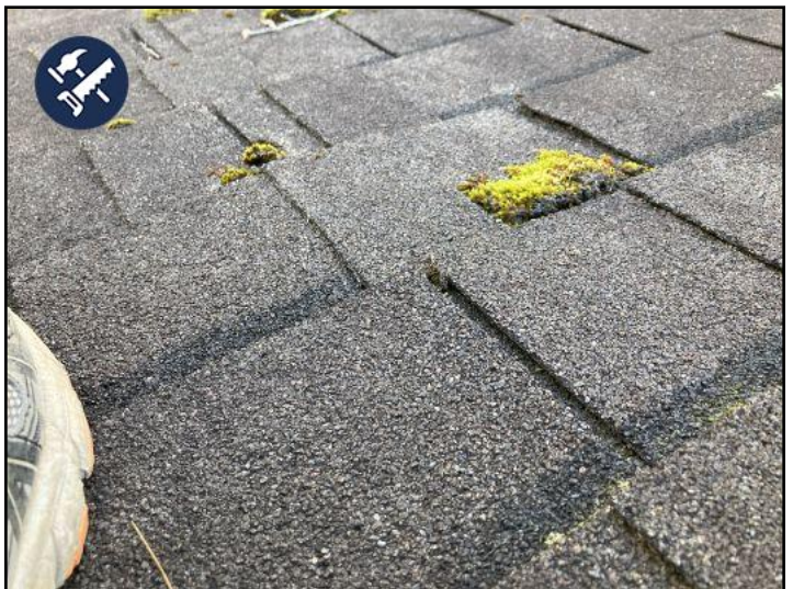
moss on the roof will shorten an asphalt shingles lifespan. Recommend spraying a fungicide on the affected areas every couple of years.
