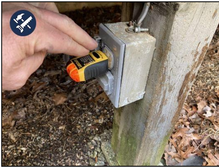
not GFCI protected.
